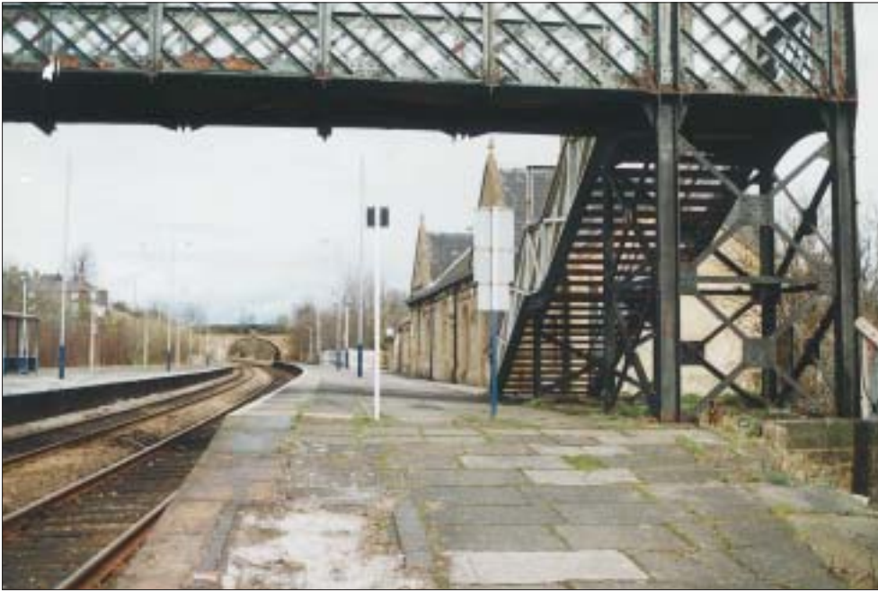
Left: looking towards Wrexham. The bus shelter has been temporarily replaced by a Portakabin until a start is made on a replica of the original island platform building.
